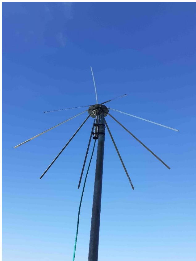
Figure 17 – Testing of the self-built ground plane antenna.
